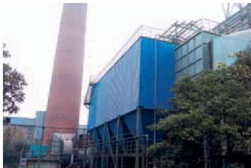
1#Sintering machine tail dust removal efficiency enhancement
